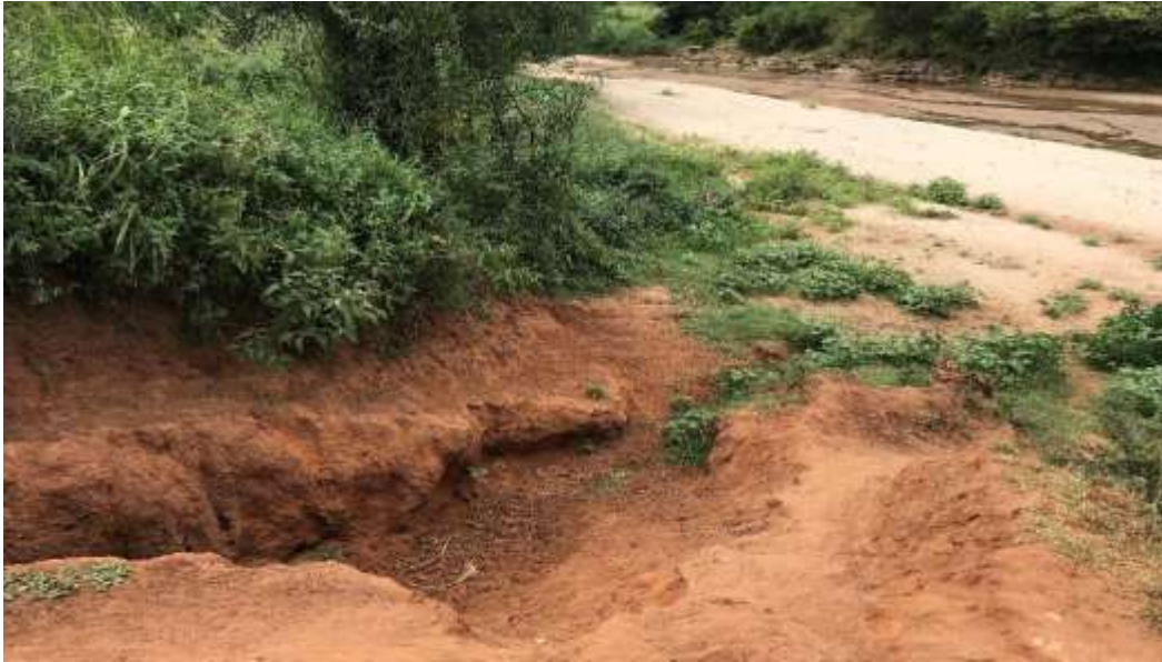
Plate 4.1: Kaiti River eroded river banks at Mwaani section
