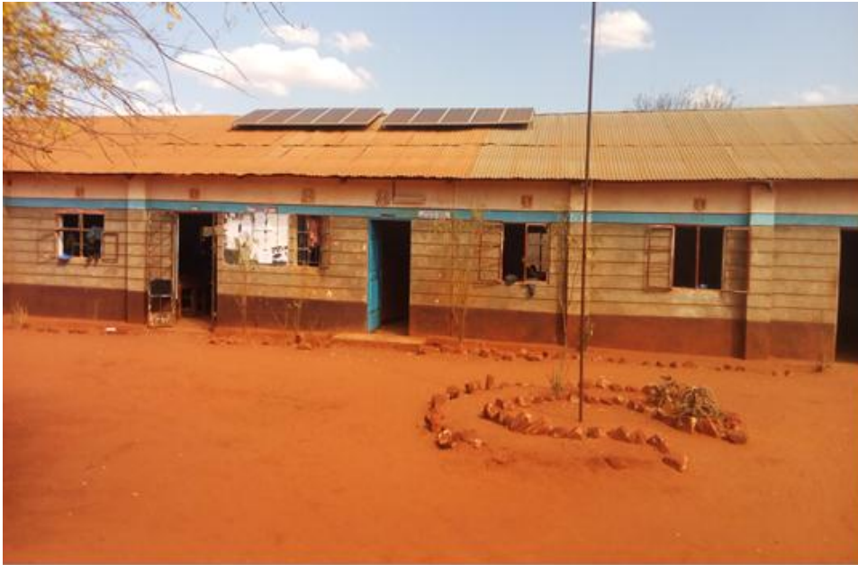
Plate 4.2: Solar panels fitted on rooftop of Yikitaa secondary school building
