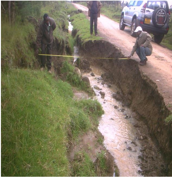
Plate 6: Gully erosion on Roads –Turasha
