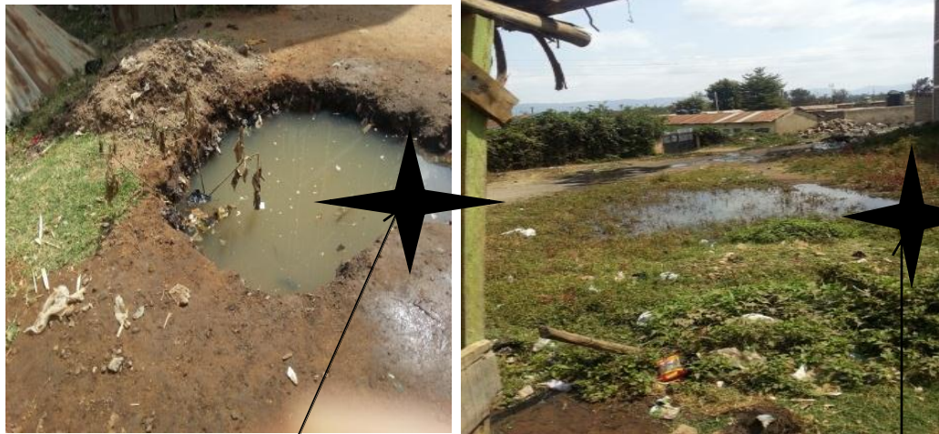
Figure 4.4 pool of water caused by leaking pipe. Figure 4.5 leaking pipe,
